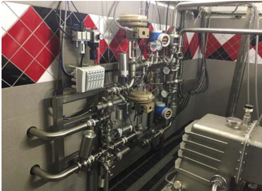
Figure 2: Valve terminals can be mounted in the open, close to the process valve actuators for faster response time. (Source: Avery Brewing)
