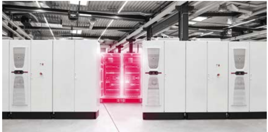
Figure 6: Many data enclosures and components such as climate-control units are now equipped with sensors that generate a continuous flow of data that is used to offer service and energy-management activities as required during ongoing operation.
