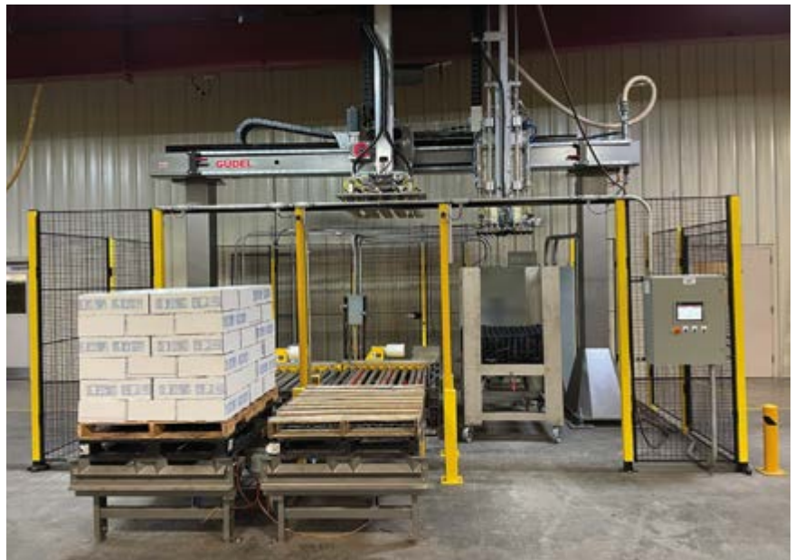
Figure 1: The gantry palletizer is a system designed for poultry processors so they can stack boxes of frozen chicken separated by special dunnage that allows air flow through the stacked boxes to assure the meat in the center of the pallet will be frozen completely. It is being marketed and sold as a pre-engineered system.
