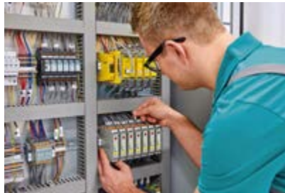
Figure 1: Miniaturization saves a measurable amount of money. We will continue to see a push for smaller and smarter control cabinets.
