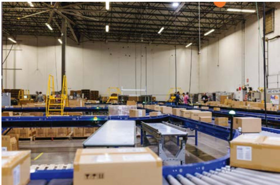
Figure 1: CTDI is increasing warehouse automation capabilities to meet demands, especially at peak times, in its global distribution centers. (SOURCE: FOREWORD LLC, 2022)
