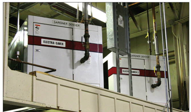
Two smaller compressors often are less expensive to run than one larger compressor
