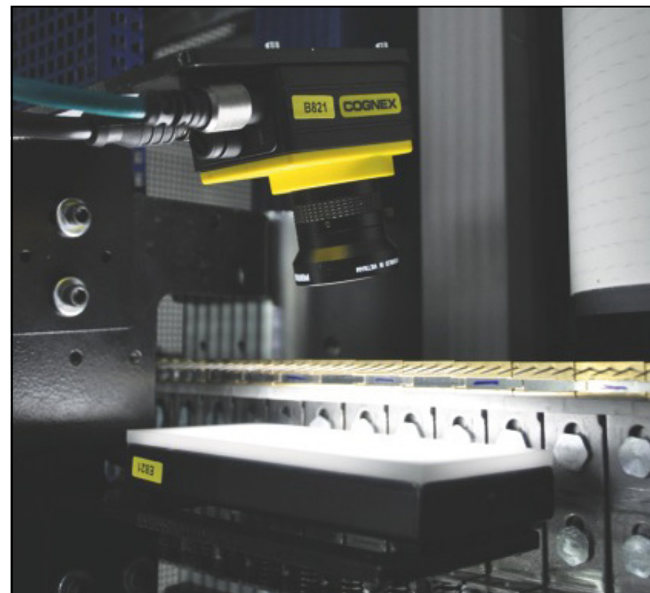
Connecting your home over the Internet to your smart phone may be revolutionary, but for industrial processes, IoT has been going on for over a decade. Here, a vision system is connected via industrial Ethernet to an Internet enabled controller.
