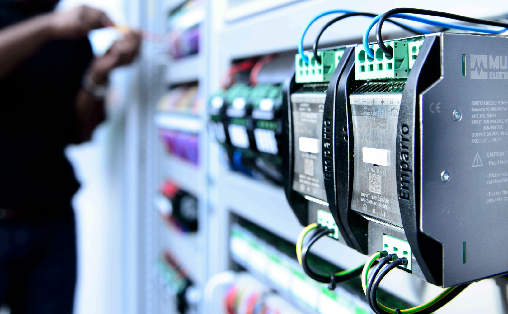
Figure 1: Control circuit power distribution is a relatively mature field, but new devices and installation practices can provide many advantages.
